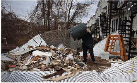
■ A home damaged by Superstorm Sandy in 2013 in the Staten Island borough of New York City. Photograph: John Moore/Getty Images
